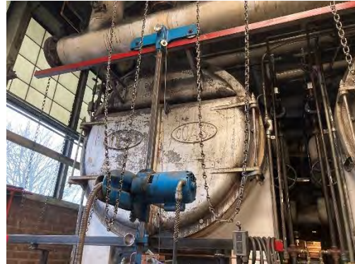
Figure 3 – Steam boiler at George Middle School.
