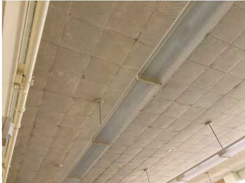
Figure 2 – Classroom ceiling in Cleveland High School.
